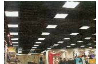
L.E.D. ceiling panel in commercial building
