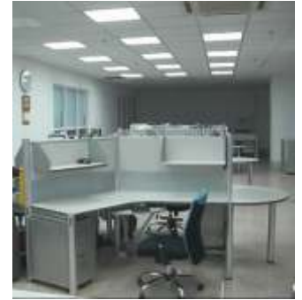
L.E.D. ceiling panel in typical office
